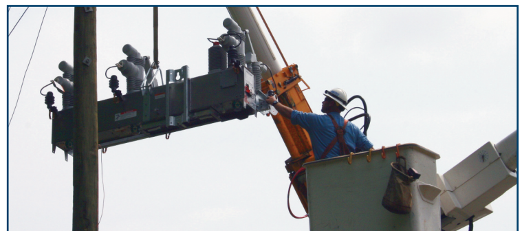
Construction Working Foreman Steve Craddock installs an IntelliRupter on the BTES electric system.
